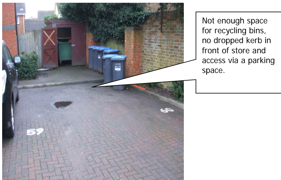
Photo 5. Example of bad practice – no drop kerb and potentially inaccessible bin store.
