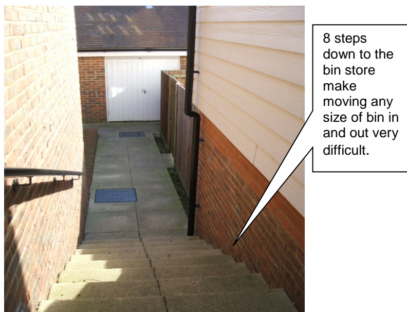
Photo 6. Example of bad practice – bin store accessed via steps.
