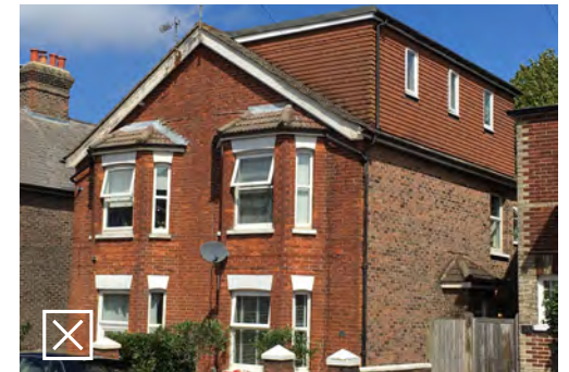
This over-sized dormer undermines the shape and symmetry of this gable frontage.
