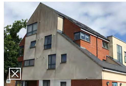
Render façades often do not age well unless they are well maintained
