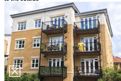
Balconies are inappropriately dominant on the façade and appear to be bolted-on
