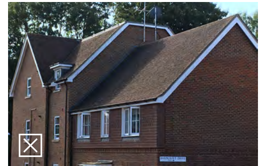
Crown topped roofs should be avoided particularly where they are visible from the street
