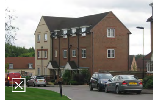
Little thought has been given to the positioning of rain water pipes, which is especially an issue when the eaves line is broken
