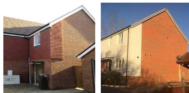
These two images show poor examples of cladding which does not continue around the first floor – uncharacteristic and inappropriate in the High Weald
