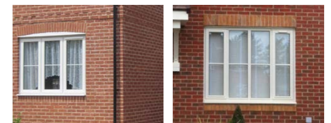
Brick arch over window and inappropriate soldier course
