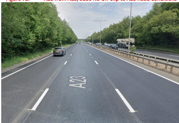
Figure 72. A23 from A23/B211 NB On-Slip to A23 Road Conditions
